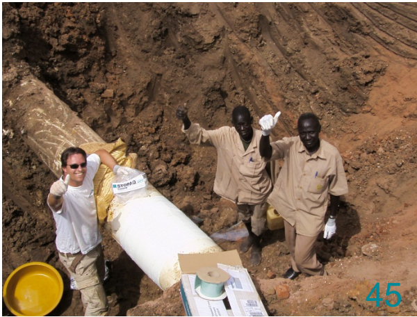
Backfill with clean sand. Backfill is possible immediately after the Outerglass Shield XT has cured.
